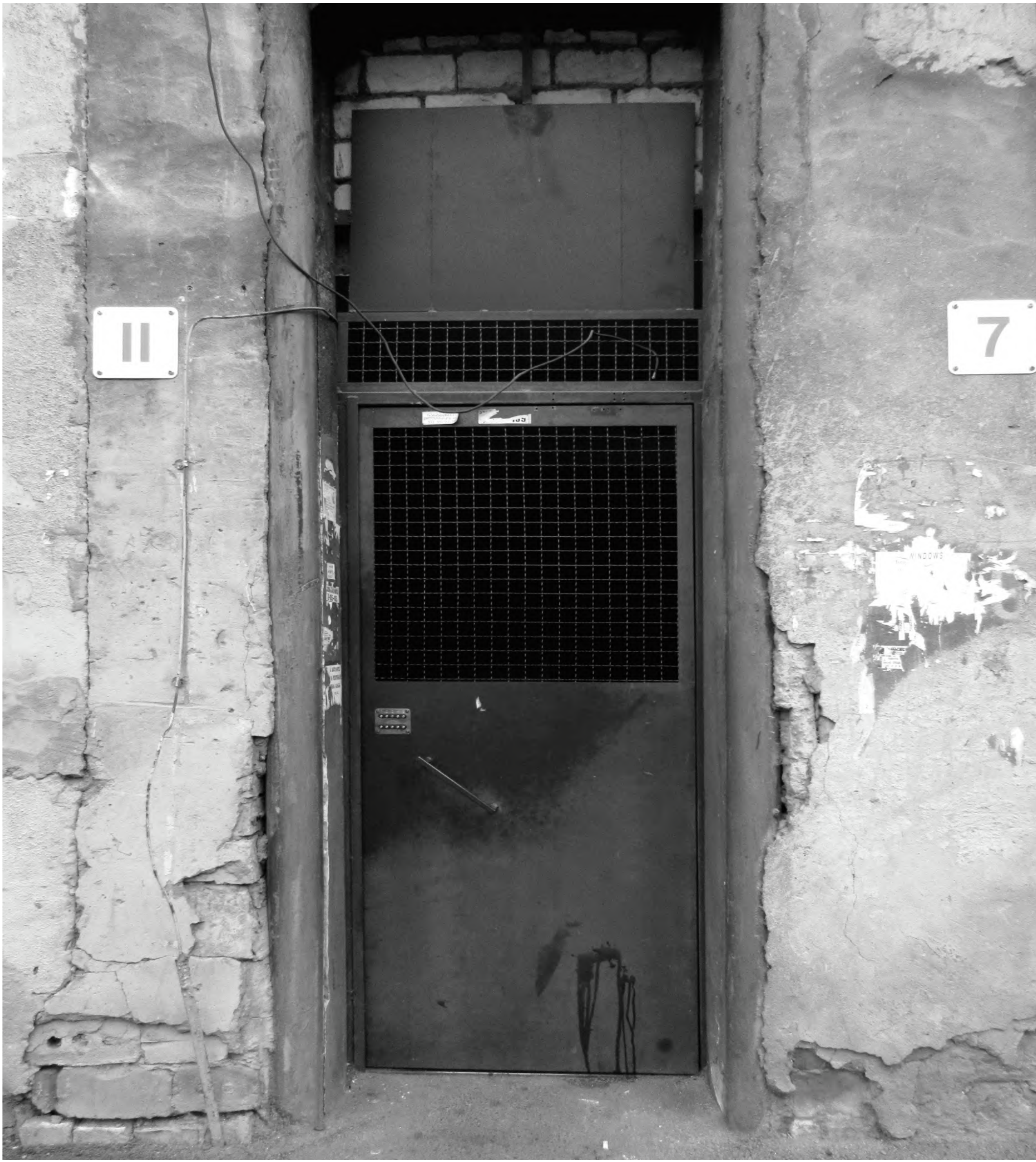
An iron door with security code secures a residential building entrance from non-residents (Saburtalo neighbourhood)
